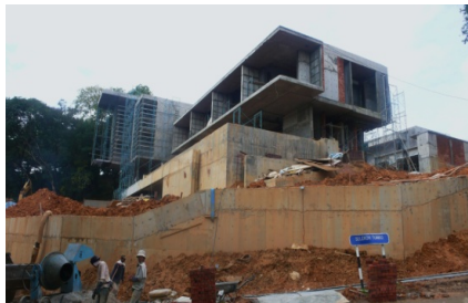
SELEKOH TUNKU HOUSE Serious earthworks and concrete slabs here. Looks like the makings of a modern masterpiece worthy of inclusion in Wallpaper* mag. The views will be stunning.
