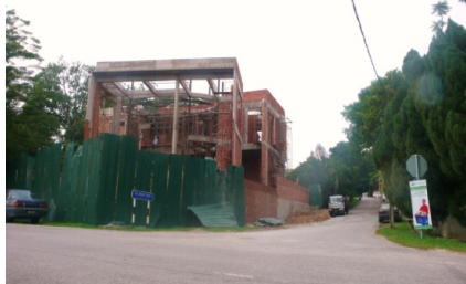
DALAMAN TUNKU HOUSE Plenty of rooms with a view in this up and coming construction in the heart of Bukit Tunku
