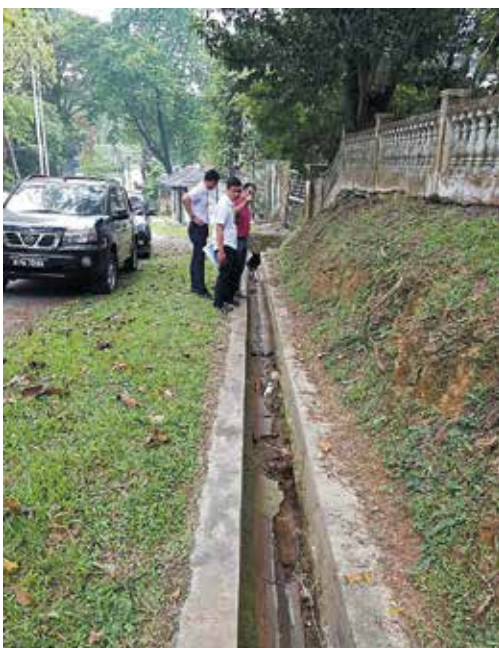
Joint inspection of drains on Dalaman Tunku by BTRA Environment Sub-Committee members and DBKL officers
